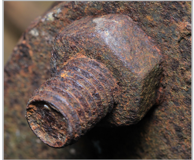
Corrosion of a nut and bolt
